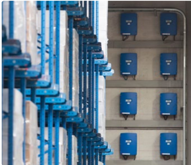
Solar panel controllers at Ieper Personal Care factory
